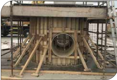
Manholes for Sewer and Drain
